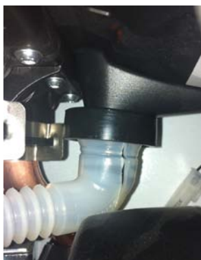
Defective siphon connection pipe.
